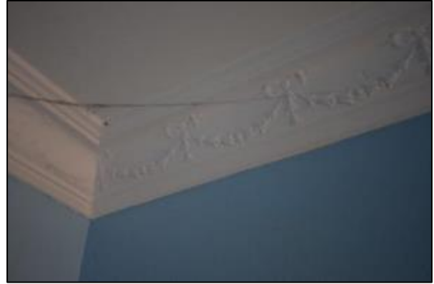
Figure 54. Original cornices in the main hall on first floor, 697 Darling Street (Source: Heritage 21, 30.11.17)
