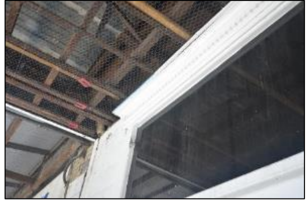
Figure 48. Detail of timber architrave and awning on original shop front on 697 Darling Street (Source: Heritage 21, 30.11.17)
