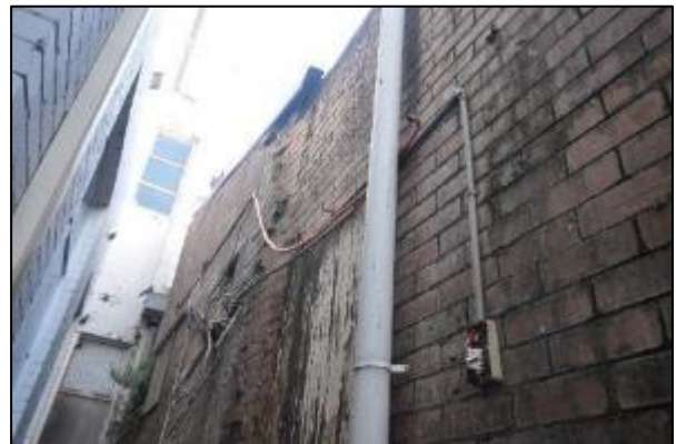
Figure 52. The rear alley with a view to adjacent building on 697 Darling Street and the first-floor window on 697 Darling street (Source: Heritage 21, 30.11.17)
