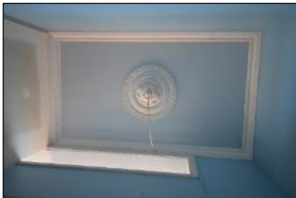
Figure 57. Original ceiling rose and cornices on ground floor lobby, 697 Darling Street (Source: Heritage 21, 30.11.17)
